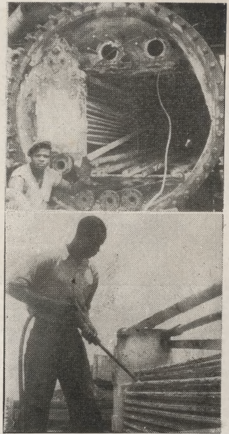
Top, Lewis Richardson uses an air-hammer to remove scale from a tube bundle at No. 2 Evaporating Plant. Below, the interior of one of the five evaporators at this plant, with two of the tube bundles removed for cleaning. Clean spares are always ready, and the evaporator is out of service only long enough to replace the crusted bundles with clean ones.
